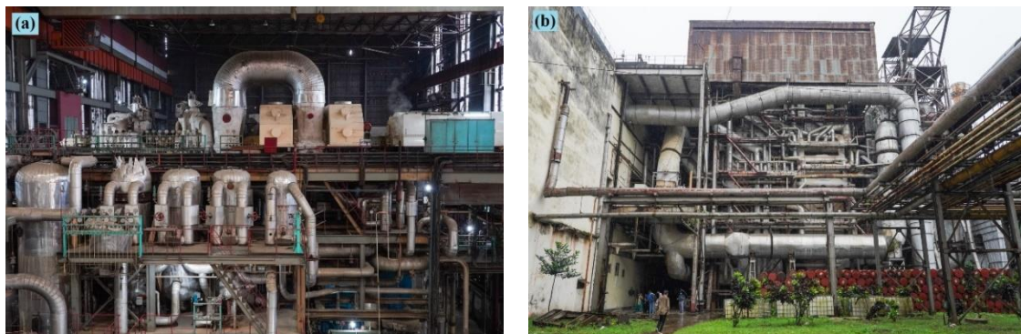
Figure 2: Ghorashal 210 MW steam power plant (a) Interior view of turbine–generator hall, (b) Exterior view of the boiler, deaerator, and main steam/feedwater piping system [28].
